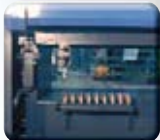
냉각수공급장치 Cooling water distributor
